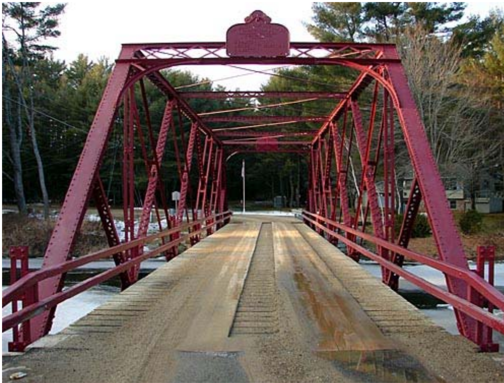
Iron bridge over Crooked River on Ryefield Bridge Road, Otisfield Gore, Maine: Photo by Bob Travis (CC)
